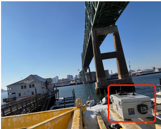
Figure 4 - Hardware Unit for Vessel Collision Warning System at Chelsea Yacht Club adjacent to the Tobin Bridge in Boston, MA
